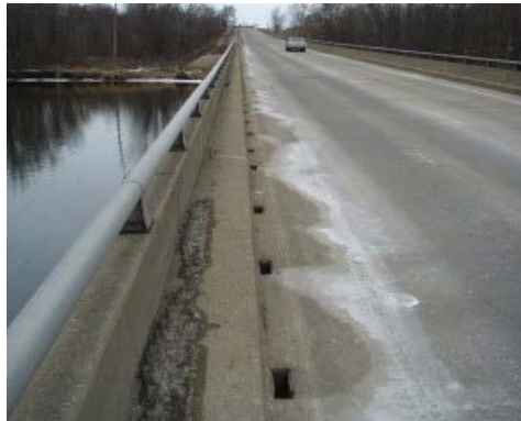
Figure 16: Salt encrusted bridge
