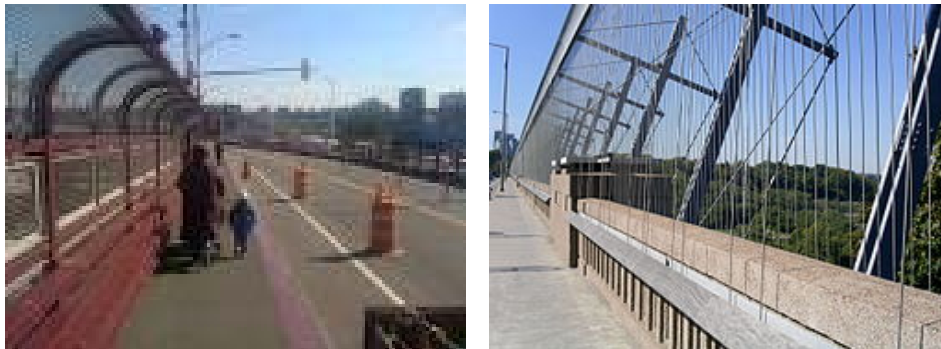
Figure 17: Examples of climb-proof fencing barriers
