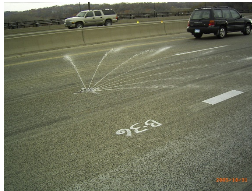
Figure 24: Bridge anti-icing system
