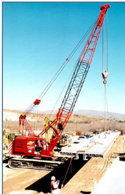
Figure 32: New bridge built with railcars. – Note that the photo shows a new bridge being building using flatbed railcars as its building component.
