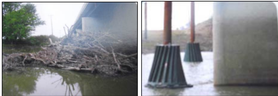
Figure 5: Debris-choked pier (left); Debris-free pier using debris shark (right)
